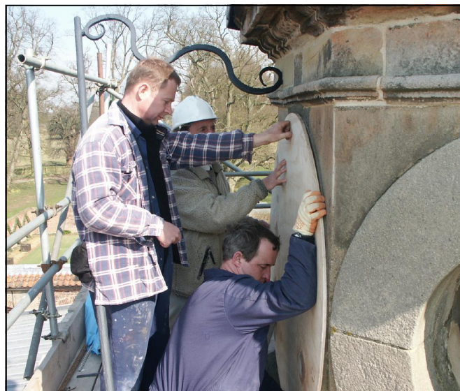
Fig 5. How many men does it take to install a sundial? Drilling the fixing holes for the plywood template of the west dial.
