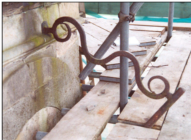
Fig 2. The top support of the "north" dial gnomon poking through the middle layer of scaffolding. Note that it meets the wall well away from the raised circular stone of the dial face.
