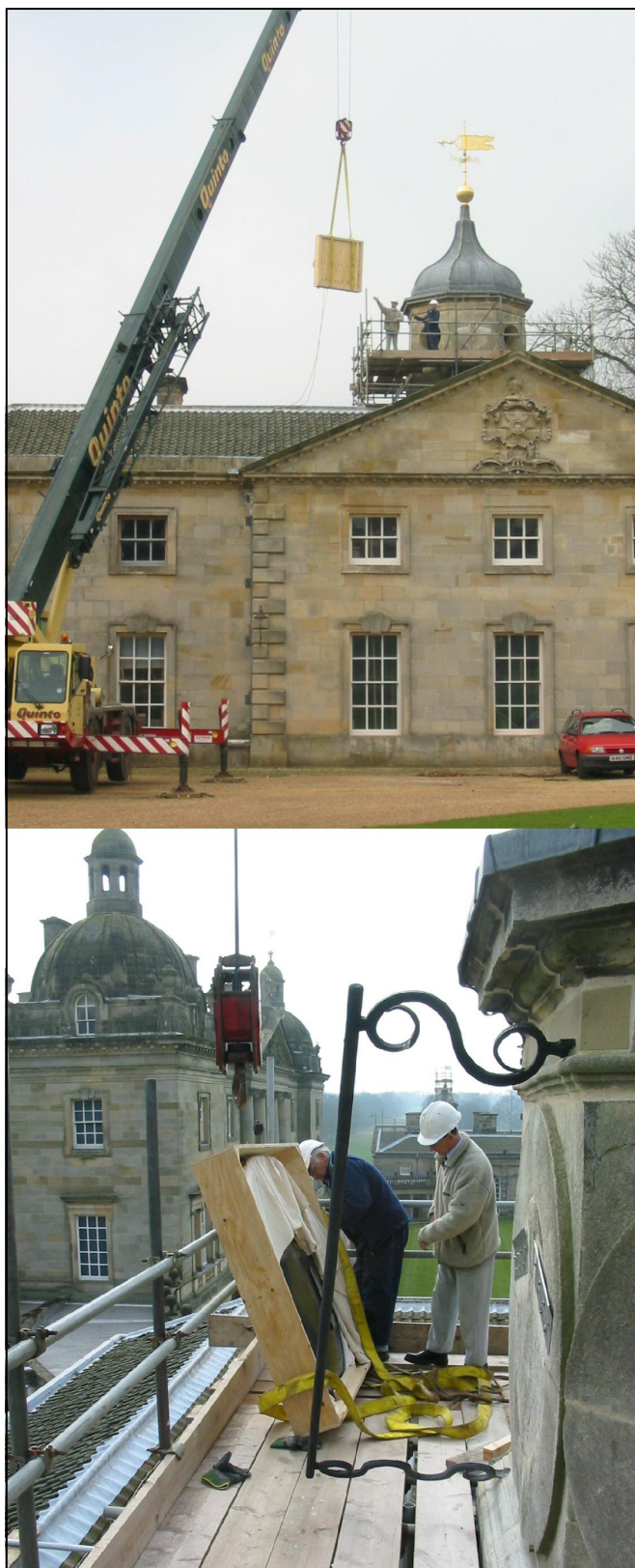
Fig 6. Craning a dial, in a protective box, onto the tower. The lower picture shows the galvanised brackets screwed to the stone to receive the dial. Photos: M. Hollingsworth.
